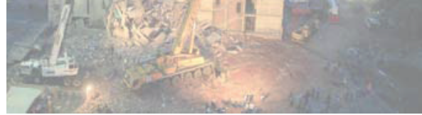
In this photograph taken on April 29, 2013, cranes operated by Bangladeshi Army personnel standing at the scene following the April 24 collapse of the nine-storey Rana Plaza building in Savar on the outskirts of Dhaka.
